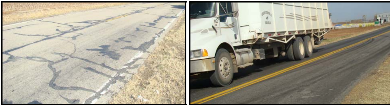
FIGURE 4. Cracking and Minor Rehabilitation
