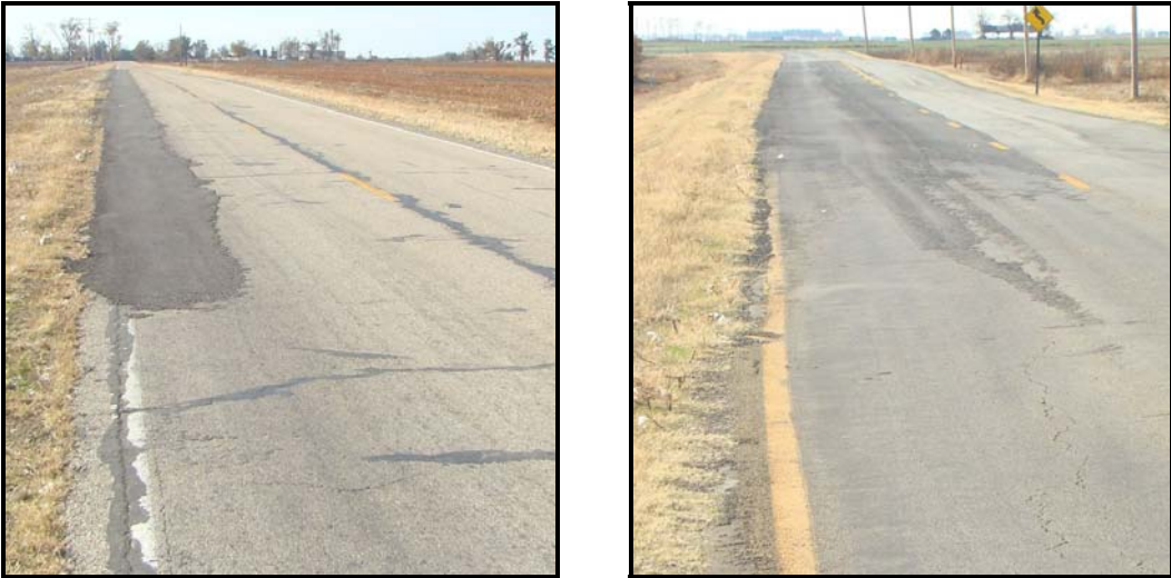
FIGURE 6. Pavement Edge Deterioration
