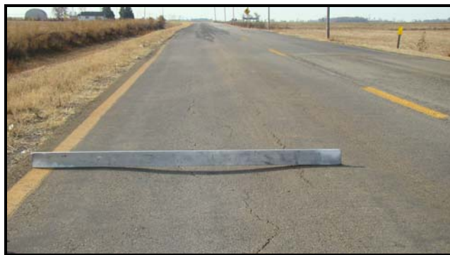
FIGURE 5. Typical Rutting Found Within Log Mile 8.4-10.46
